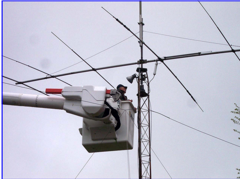
MY HERO! MARCEL-W1MLD WORKING ON THE DAMAGED BEAM.
