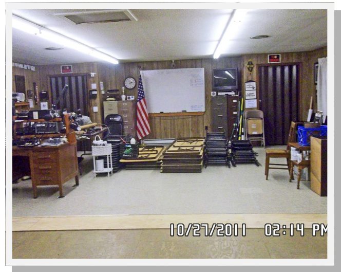
HALF THE NEW FLOOR COVERED TO ALLOW REST OF FLOOR TO BE INSTALLED
