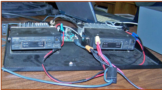
COMPLETE D-STAR REPEATER ON A RACK.
