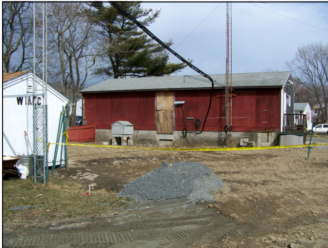
CURRENT LOOK OF THE REAR OF THE CLUBHOUSE - GROUND HAS BEEN LEVELED AND CINDER BLOCK FURNACE BUILDING RAZED.
