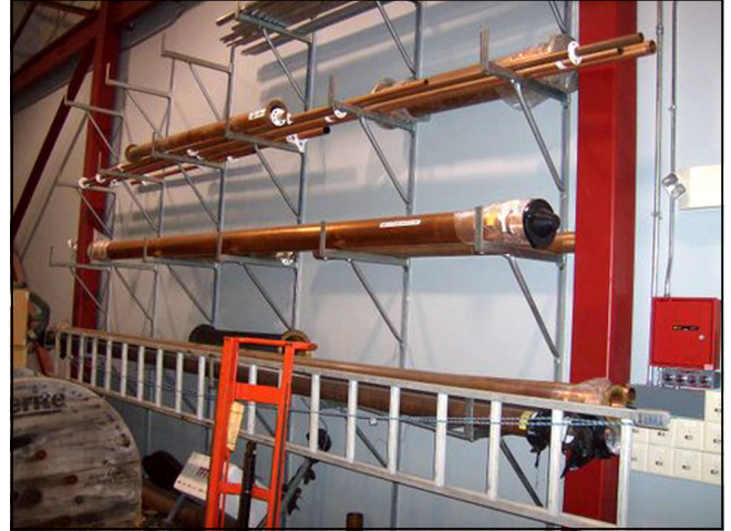
COAX SPARES ON THE RACK. (USE LADDER FOR SCALE.)
