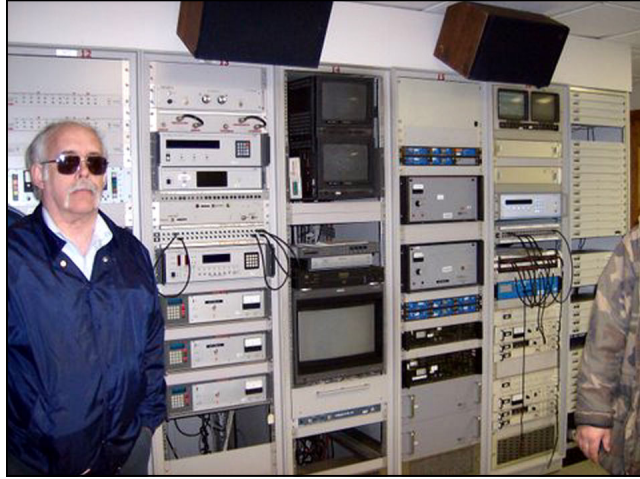
TRANSMITTER CONTROL STATION.
